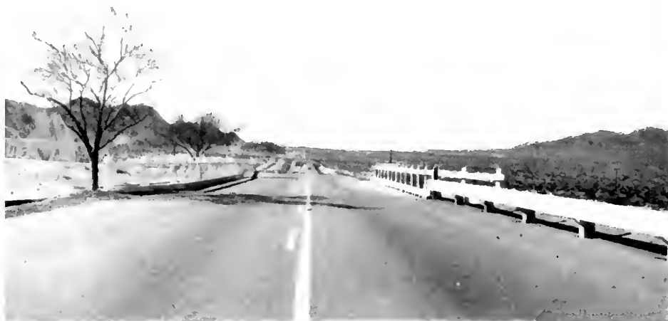
This photo shows type of flared guard railing used at bridge approach
